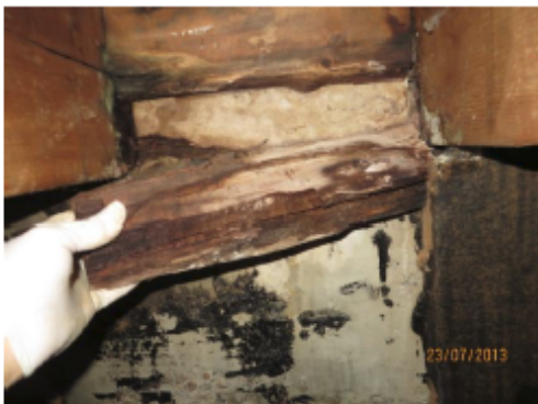
The rotten blocking was broken away by hand and was powdery with cuboidal cracking (Caused by fungi that have removed the cellulose from the wood and left the lignin, Sometimes referred to as 'Brown rot' or 'dry rot')
