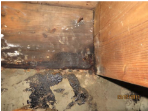
View of the left side of the central joist, note the white mycelia, and dark staining indicating fungal attack
