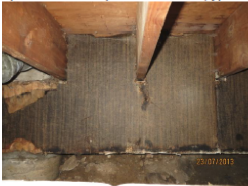
Undisturbed condition as discussed on previous page
