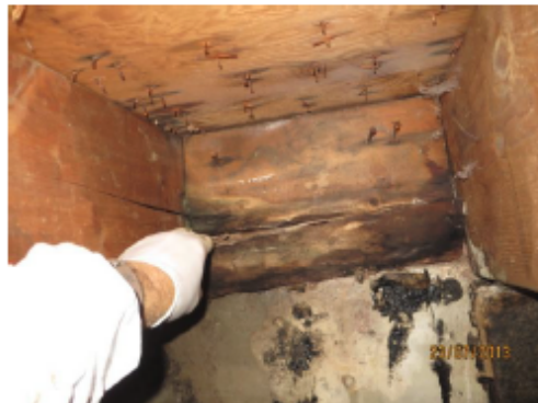
View of the right side of the central joist with a finger penetrating the rotten wood of the blocking
